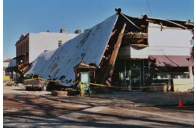
Figure 1. Collapsed Building (DHS Photo)
