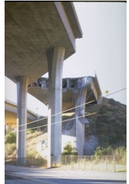
Figure 2. Bridge Destroyed by Earthquake (DHS photo)
